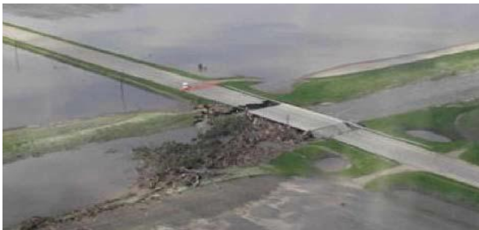
Figure 1-3 A bridge failure in Wild River, Minnesota case caused by the interrelated action of scour and debris accumulation against the structure. This is common for small bridges, where bridge openings narrow the natural channel and form an obstacle to the flow (after Ettema et al., 2006).
